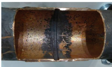
Figure 9: Brazed tube, no back shielding
