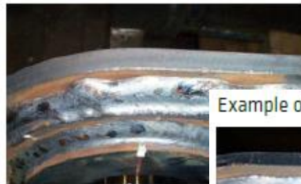
Example of bad wire placement
